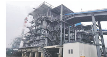
国能泊头36吨生物质锅炉 36 T Reciprocating Grate Biomass Boiler
