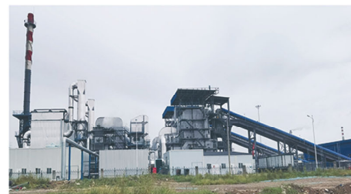
国能泊头36吨生物质锅炉 36T Reciprocating Grate Biomass Boiler
