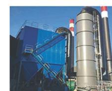
脱硫塔 Desulfurization tower
