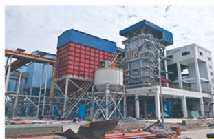
越南赛轮 75 吨燃煤循环流化床锅炉 75T Coal-fired Circulating Fluidized Bed Boiler in Vietnam
