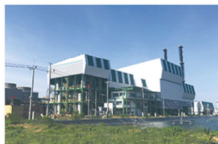
泰国酿酒厂 2x30 吨棕榈壳锅炉 Two 30T fired Palm Shell Boilers in Thailand
