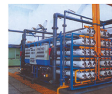
反渗透 RO System
